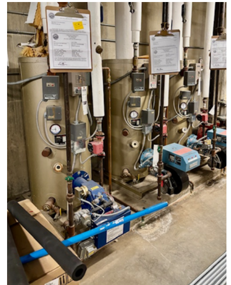
Old Boilers in Basement
